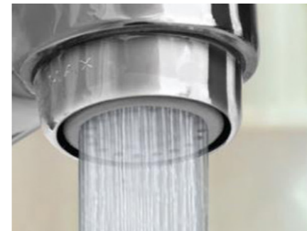
Faucet Aerators Faucet aerators (the wire screen where water comes out of your faucet) that are not cleaned regularly may also increase lead exposure. Periodically remove debris from faucet strainers – we recommend twice a year. Remove the strainers/screens from the faucets you use for consumption, rinse off the strainer, and run the water for 3 to 5 minutes.
