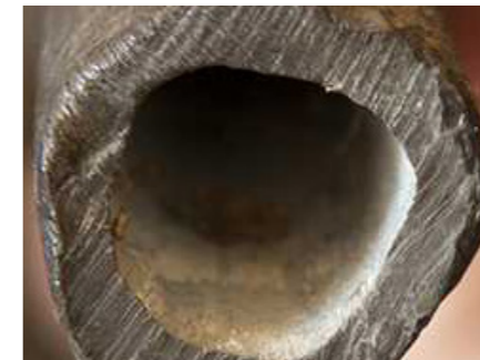
Lead In Pipes Some lead may dissolve into water when water sits in your pipes overnight or when it is unused for several hours during the day. As a precaution, let the cold tap water run until you feel a change in water temperature to make sure you're getting water from the main in your street. This usually takes 30 seconds to 2 minutes. This can minimize the potential for lead exposure in water used for drinking or cooking.
